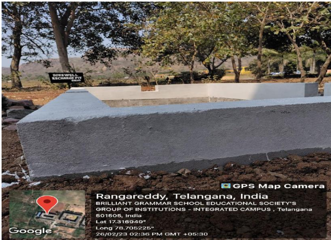
Bore well recharge pit.
