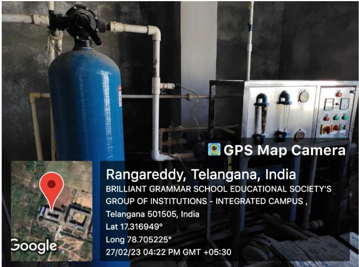
RO water plant.
