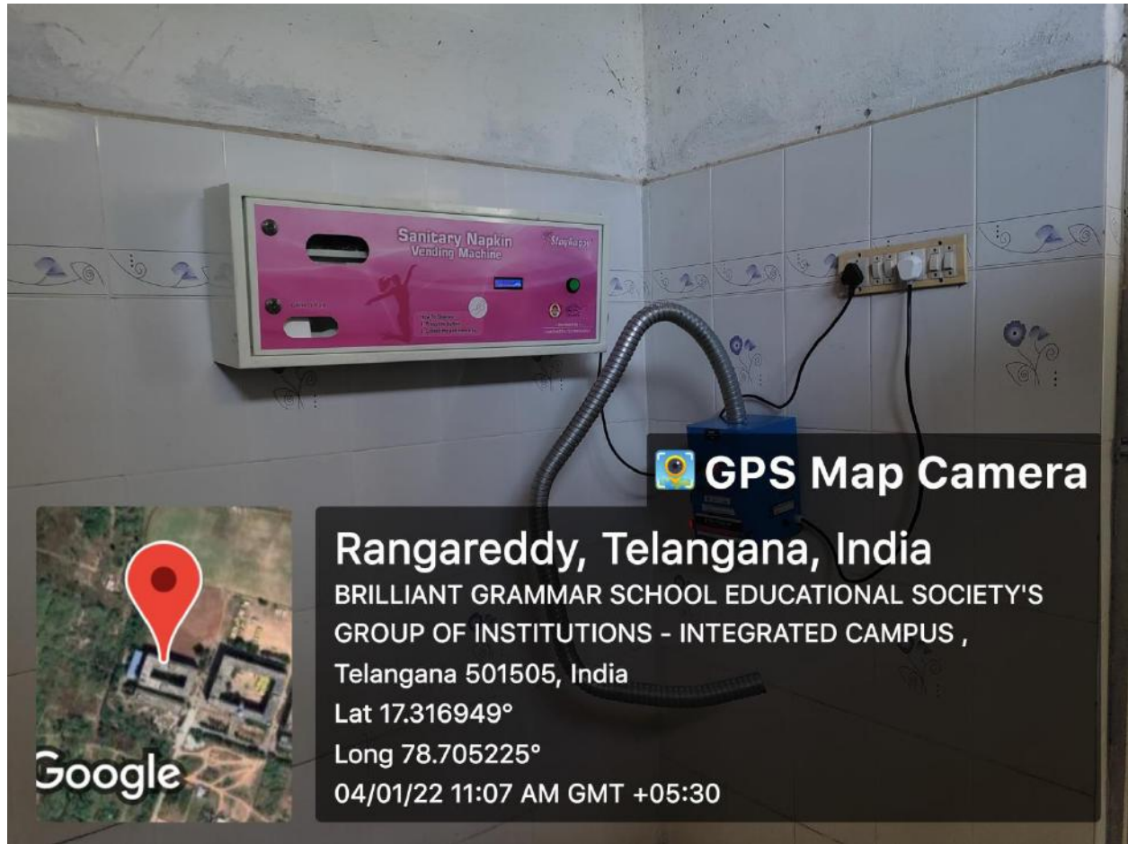
Vending and burning machine in the institution premises
